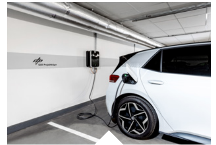
E-charging station of DLR-PT at Godesberger Allee 138 in Bonn
